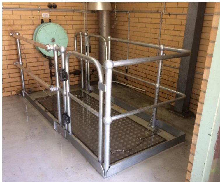
Figure 6: Example of aluminium covers with permanent guard rails inside a building. (Note: a ground level standing area in front of the ladder inside the guardrail area has not been provided in this example but shall be provided if practical. Refer Figure 1)
