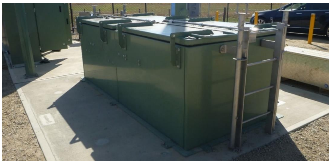
Figure 11: Example of turret top close up (note: missing rubber door stoppers)
