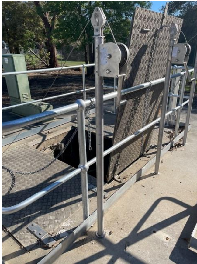
Figure 4: Example of winch set up for fabricated metal covers > 20kg in weight. An in-ground sleeve located behind each cover is with a single mobile post and winch is acceptable in lieu of multiple fixed winches
