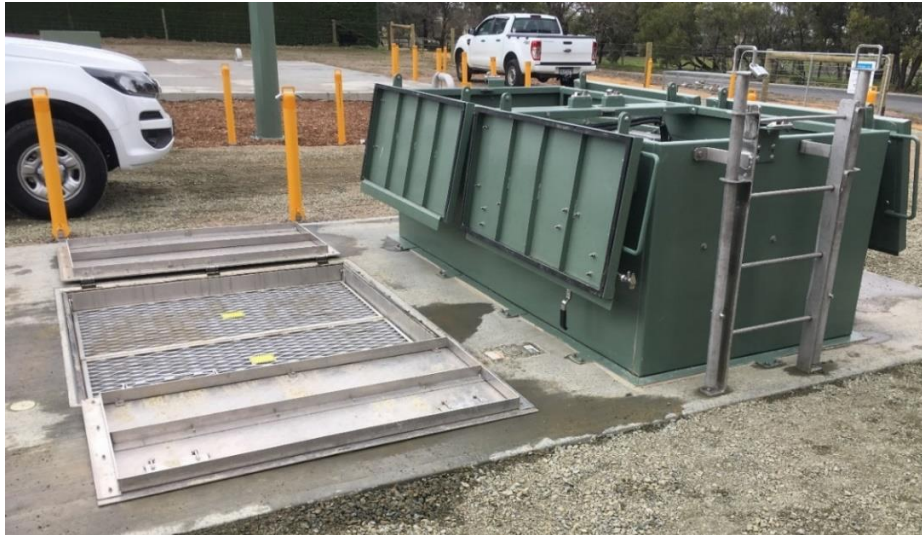
Figure 12: Example of turret top opened-up (next to aluminium covers opened-up) (Note that fabricated metal covers shown are not compliant)
