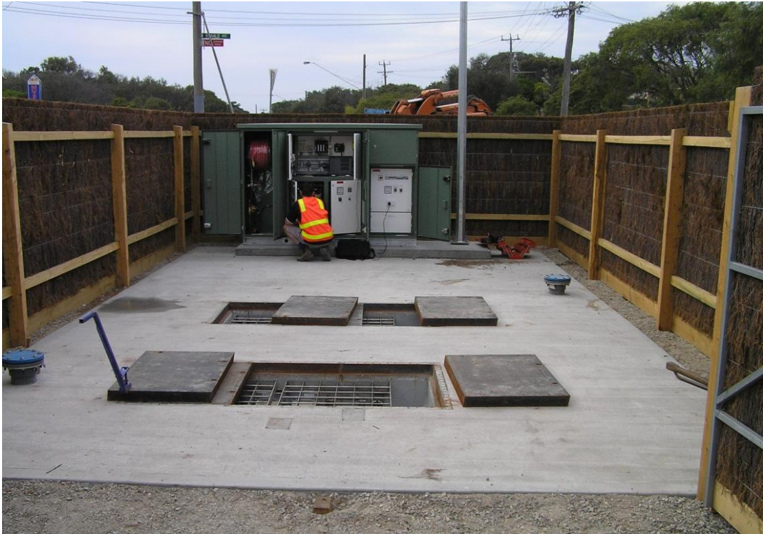
Figure 10: Example of Multipart trafficable concrete infill ductile iron covers (Guard rail system not yet installed)
