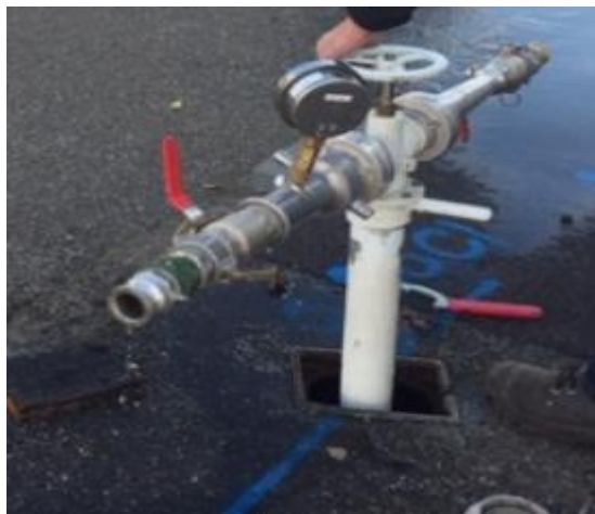
Figure 2 Incorrect hydrant test set up
